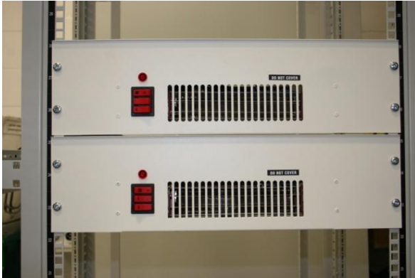
Heat Load Unit – Rear Exhaust
